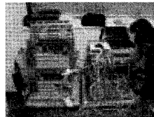
Core routers (Juniper M20). And Router testers
