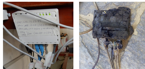
Figure 3 Damage caused by Lightning at Deurali
