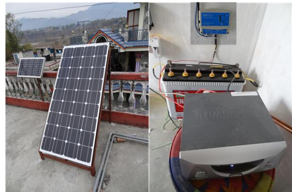
Figure 2 Solar Backup System in Pokhara Station
