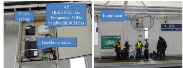
Figure 5: Snapshots of installed equipment at a station.
